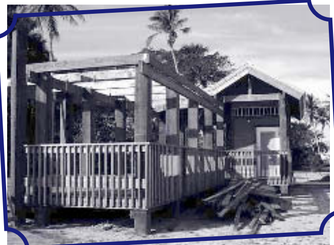
Work on the first phase of the RRC's education pavilion was nearly completed in February when this photo was taken (photo by John Worth).
